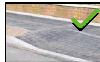
Uninterrupted footways over driveways
