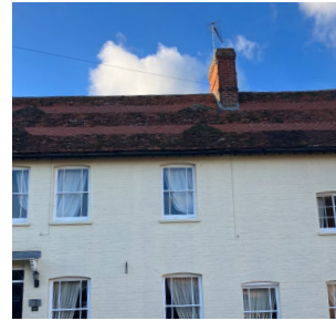
Light red colour fishscale band detailing on a dark clay tile roof
