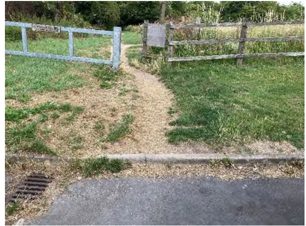
Kerb at the end of Ivel Way
