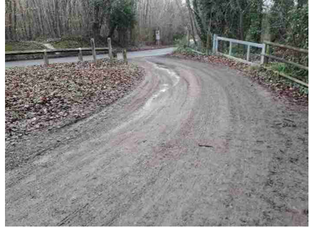
Rutted entrance to Chalk Hills car park
