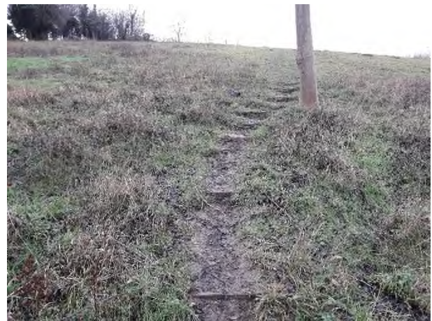
Dilapidated steps on Gibbet Hill
