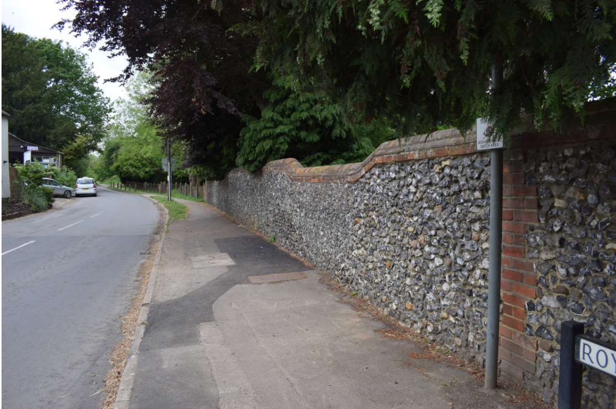
Figure 2.2 An example of brick and flint boundary walling, this section being on Royston Road (looking west).
