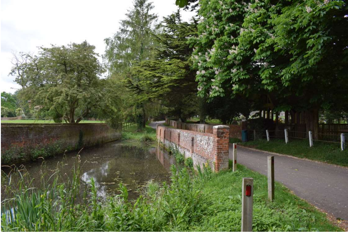
Figure 2.3 The wagon wash, a distinctive structure related to Barkway's history as a stopping point a coaching route, which was used to clean coach wheels and name plates (looking west).
